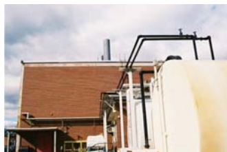
Rowan University's Cogeneration Facility.
