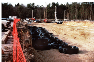
The Geothermal well field being installed at Richard Stockton College of New Jersey.
